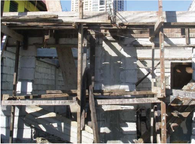
Example of construction in a Gawad Kalinga village in Metro Manila. The use of masonry concrete units is dominant even if the life cycle of these structures is short. Gawad Kalinga Village, Metro Manila
